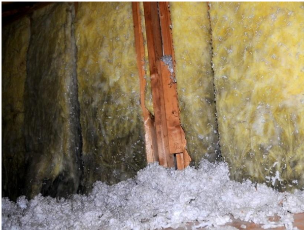
Pic 8: Mold growth on Insulation.
