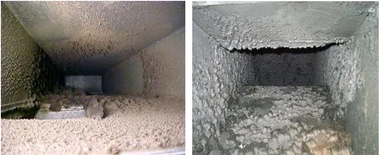
Pic 4: Mold growth inside duct.
