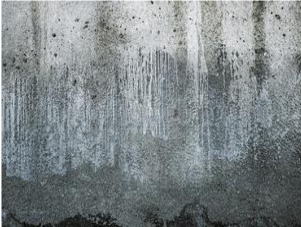
Pic 7: Mold growth on concrete surface.
