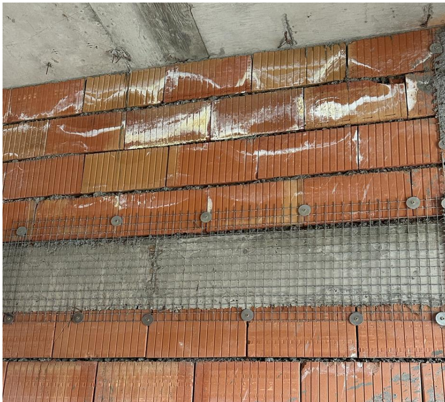
Pic 14: Efflorescence on brick.
