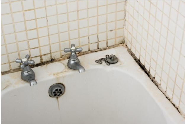
Pic 11: Mold growth on tile.
