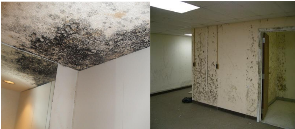
Pic 10: Mold growth on painted surface.
